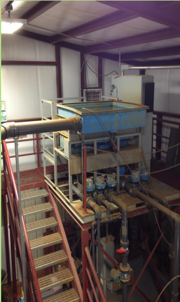
50 gpm Tertiary Treatment Oklahoma WWTP
