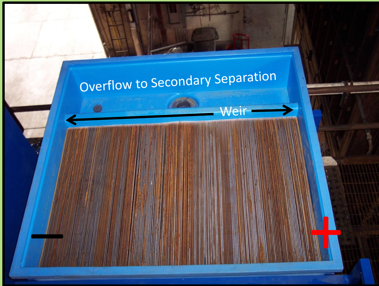
Central Wastewater Treatment Facility (CWT) 50 gpm, Denver, Colorado
