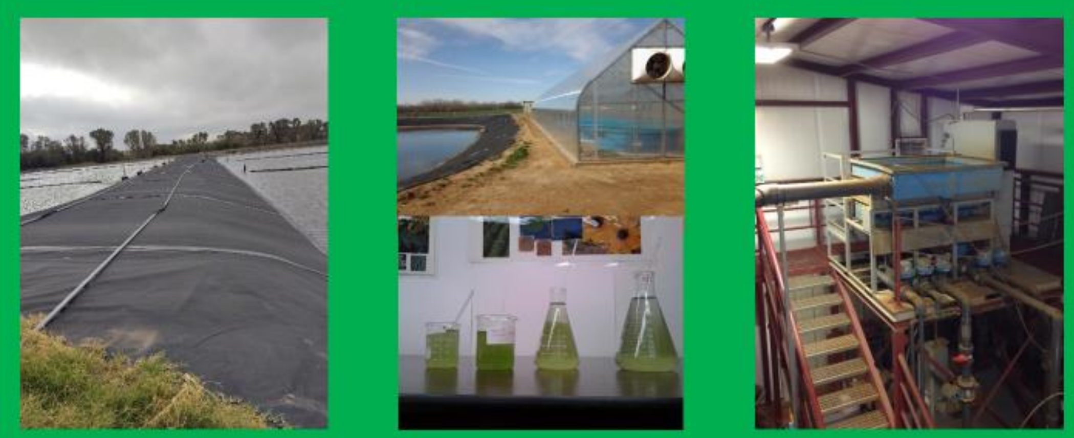
Primary Treatment Lagoon efficiency improves with additional oxygen. Selected micro algae and microbes allow nature to clean the water for reuse. Tertiary Treatment Removes heavy metals, viruses, bacteria, etcetera.
